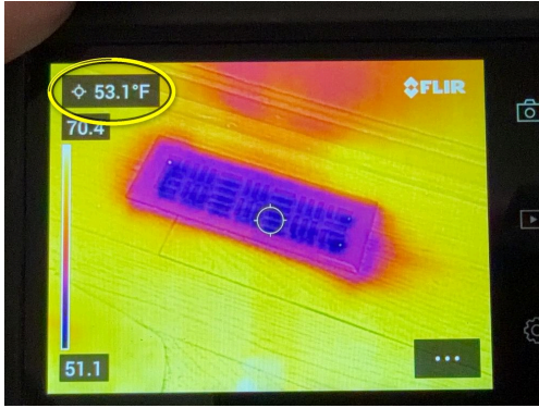
Supply air temperature
