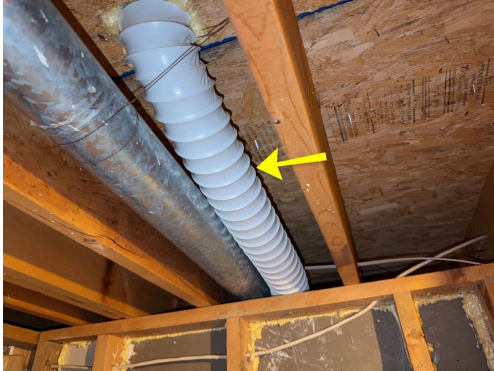
Dryer vent runs above finished drywall ceilings and basement
