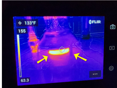
The water heater flue appears to be properly drafting during the inspection when observed with infrared
